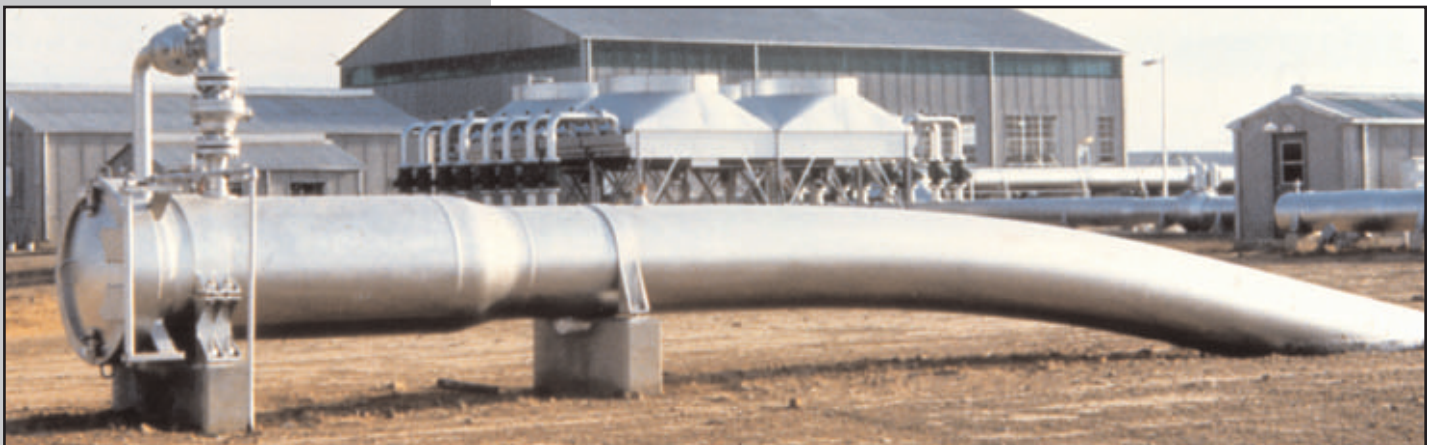
Typical of Tube Turns Yoke Type Hinged Closures being used with scraper traps.
